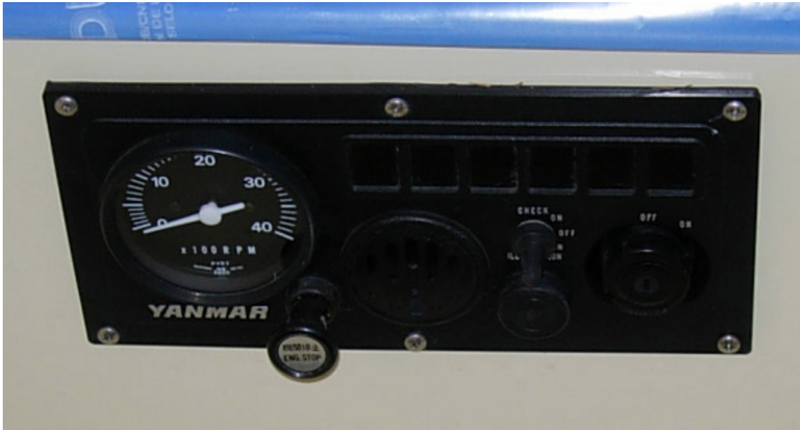
Figure 1: Original Engine Control Panel Installation
